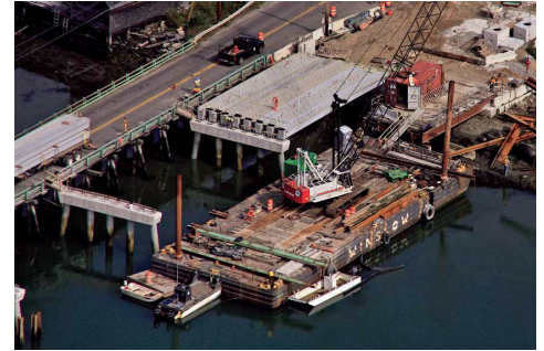
Seventy-foot-long structural hybrid bridge beams, bonded with SCIGRIP SG230 HV adhesives, are being craned into position on this causeway.
