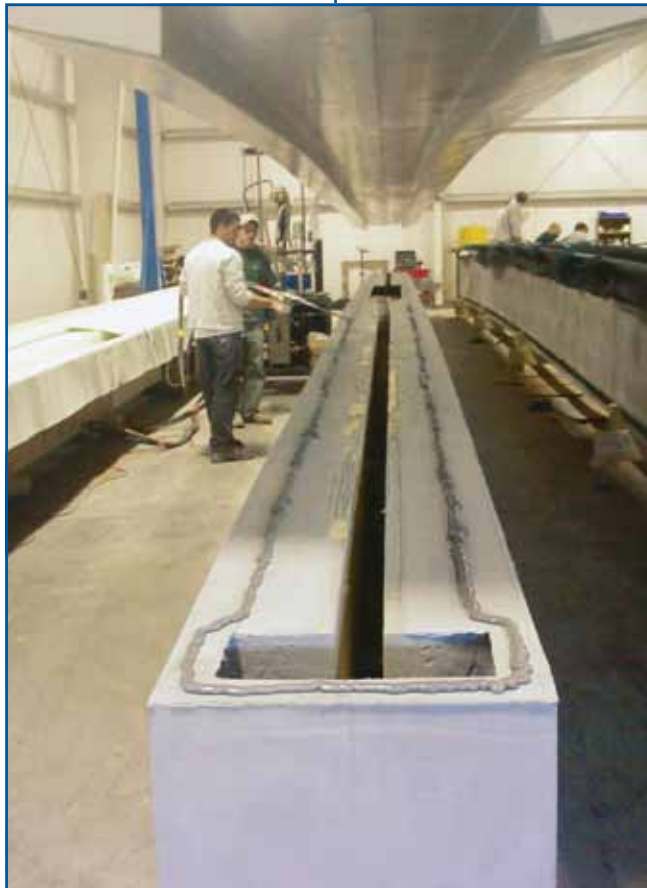
Technicians at Harbor Technologies dispense a bead of SCIGRIP SG230 HV adhesive on the composite bridge beam. The adhesive is used to structurally bond a composite top to the beam. The bulk meter-mix dispenser improved productivity by 50 percent.
